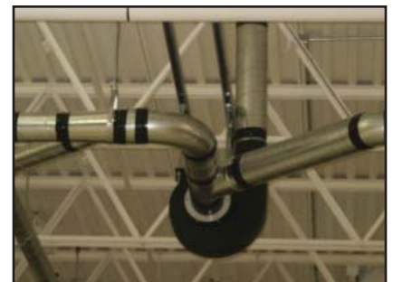
Support beam mounted
