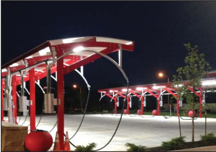
Vacuum arches under canopy structure with LED lighting
