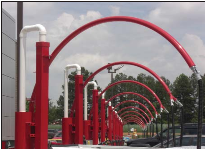
9' vacuum arches with in-ground PVC piping
