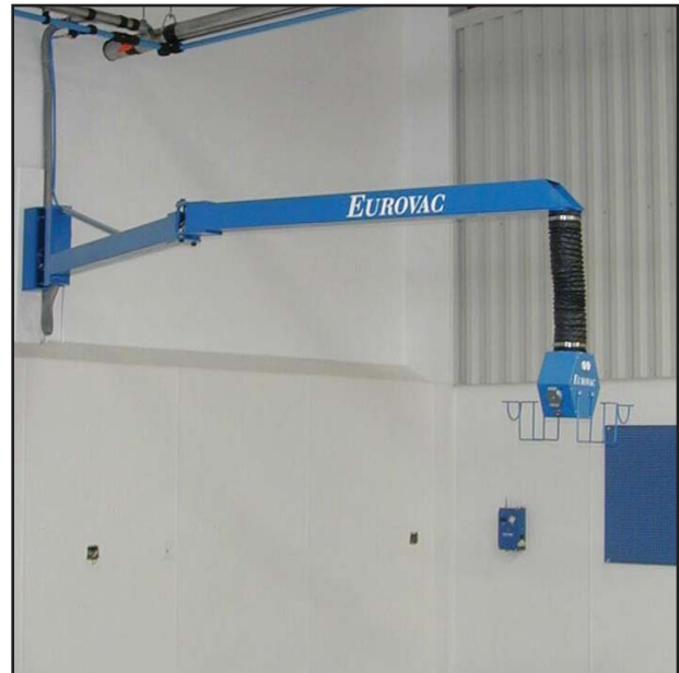
Articulated booms & pendant drops with dual inlet, integrated compressed air and 110v electric.
