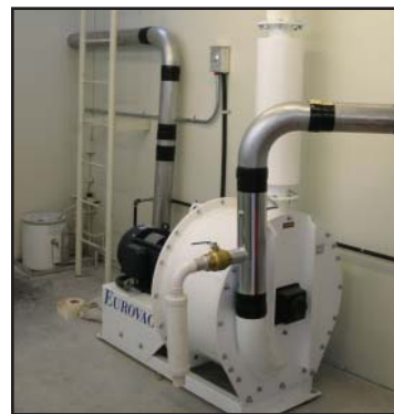
High Vacuum Turbine Pump
