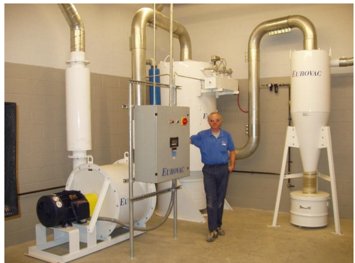
Eurovac III with PLC Control Panel
