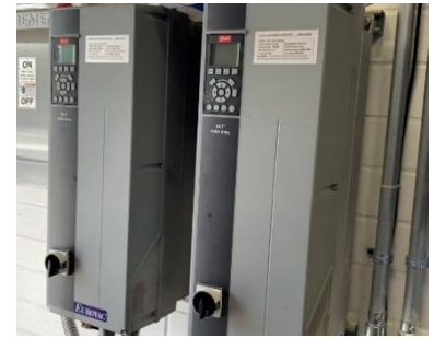
Variable Frequency Drives (VFD's)
